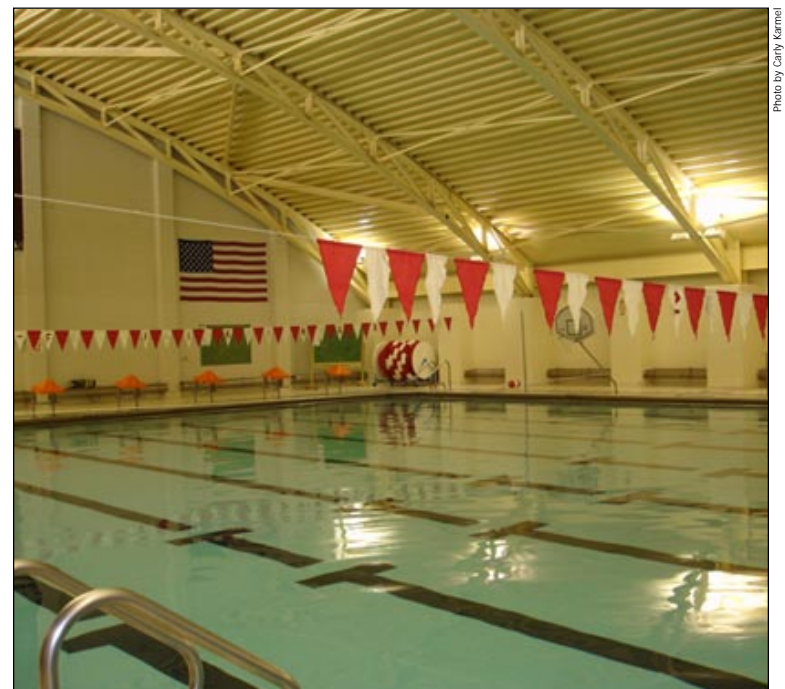
Closed no more Ever since a 50-foot-long air duct fell onto the pool area's bleachers, the surrounding area had been closed off to the rest of the public. Director of Operations and Maintenance Tom Wagner expects for gym classes to re-enter the pool next week.
